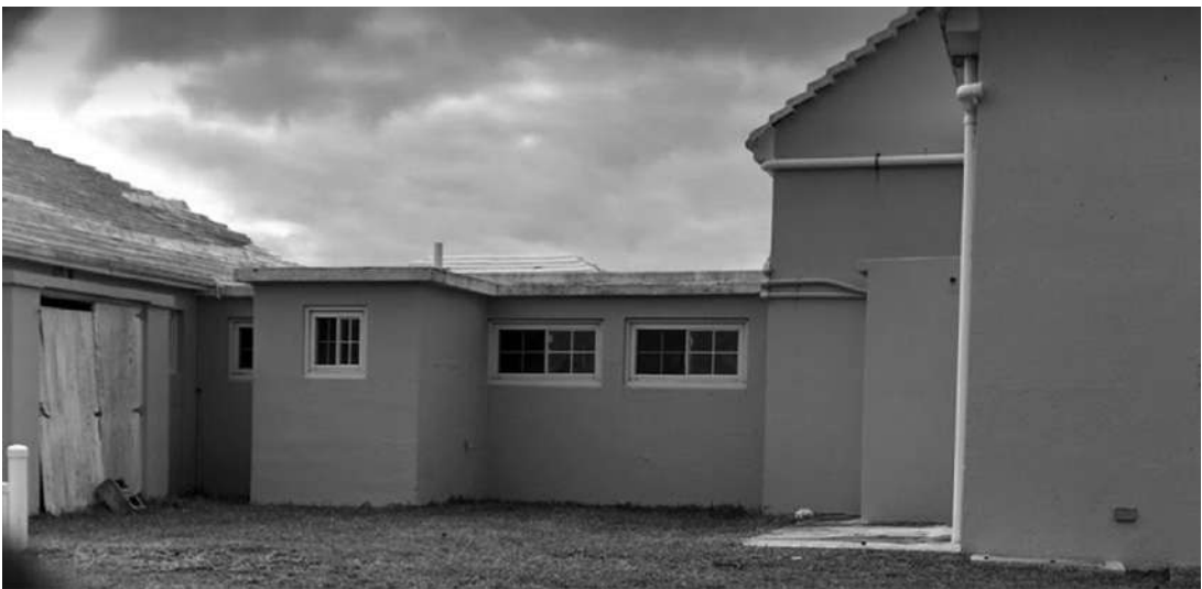
Figure 19-1 Photo of Water Collection System in Bermuda. Water is piped from roof tiles to cistern below building.
